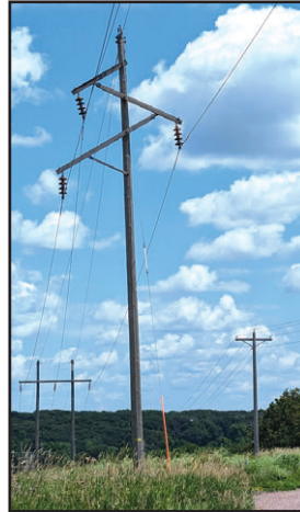
Left side: transmission line. Right: three-phase distribution pole.
