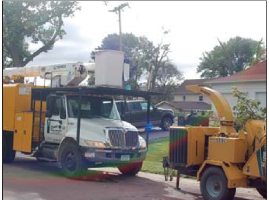
Tree trimming is like preventative maintenance. The co-op trims back branches growing into power lines before they cause an outage when loaded with ice or bending due to high winds. Let the cooperative know if branches are growing into power lines; the co-op hires Carr's Tree Service to trim trees safely near our lines.
